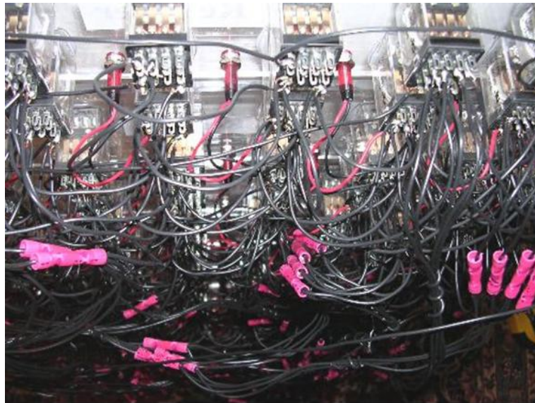
Figure 3: Mechanical switches use in industrial applications.
